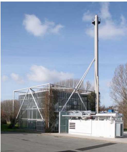
The state-of-the-art combined heat and power unit supplies Wilkhahn with electricity and heat, and results in a CO 2 reduction of 78%. Photo: Wilkhahn
